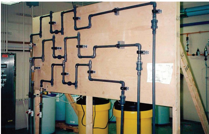
This photograph shows a pipe loop/coupon study. Source: AWWA 2011, Figure 6-8
